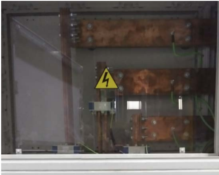
The upper module contains part of the copper busbar system along with the current transformers.
